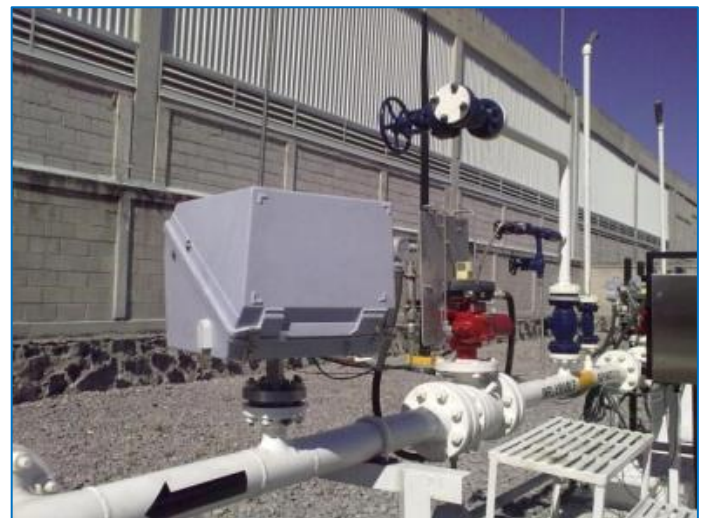
Figure 7 - Gas PTi pipeline mounted installation – Fermaca, Mexico City Business Park.
